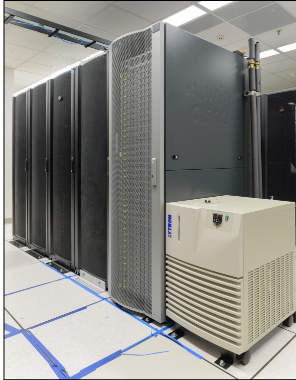
Figure 2-1: View Of Rack Containing 38 Cisco Servers Equipped With Asetek Direct Cooling Technology - Lytron CDU Shown In Foreground
